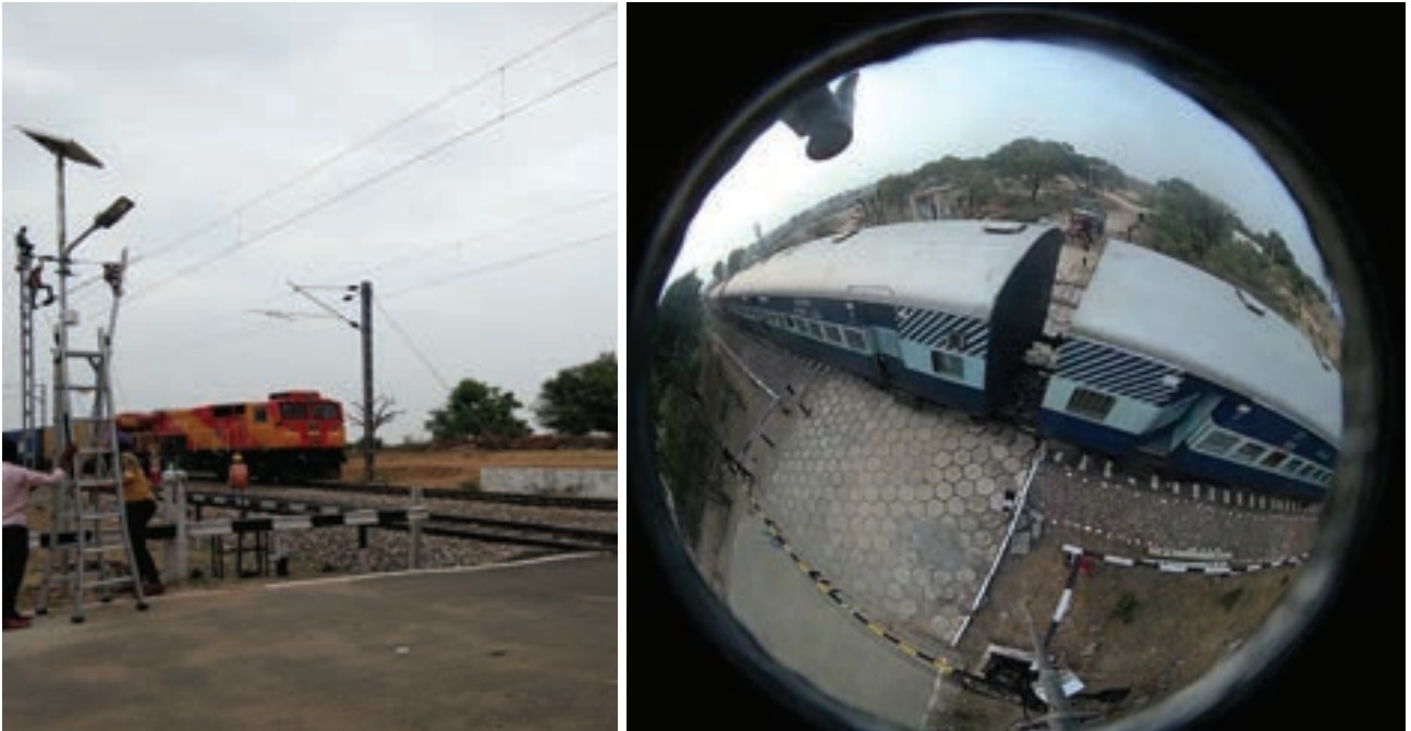
Figure 3 Solar LED street light with inbuilt CCTV at a railway crossing in Jaipur (left) and inbuilt camera vision (right)
