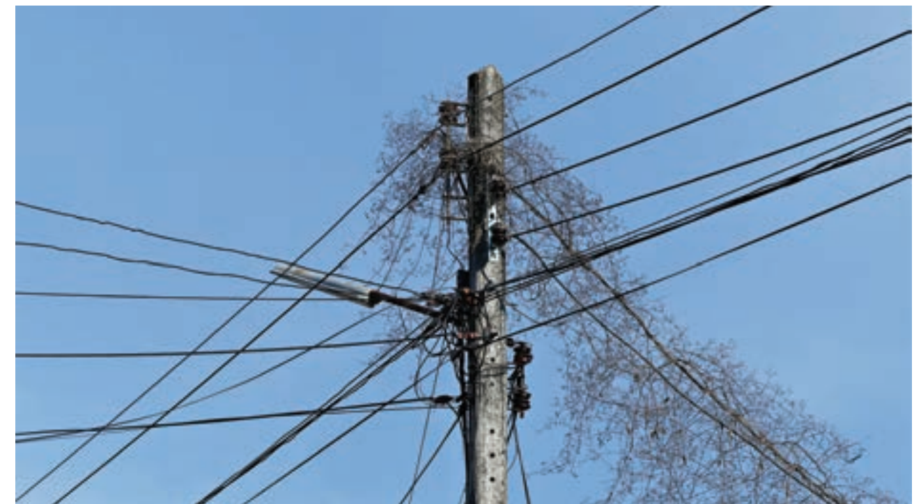
Figure 1 Expensive cabling and age-old infrastructure for grid-connected street lights
